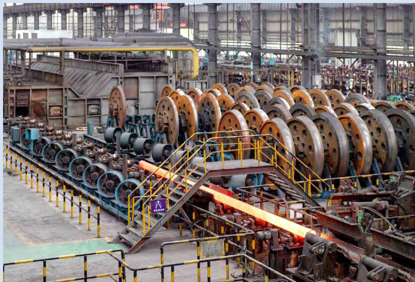
★ In-line heating furnace and guide plate
